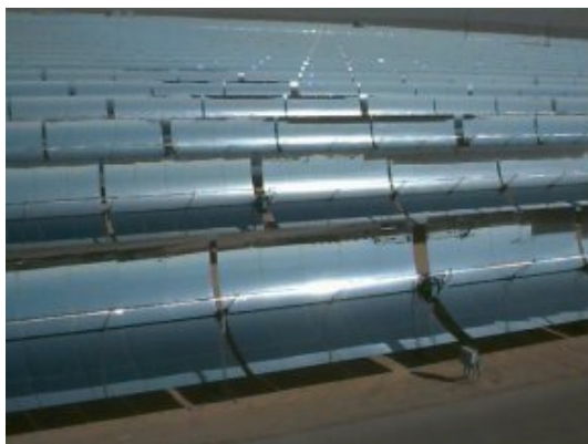
Parabolic trough power plant (Source: Stock photography (copyrighted))
